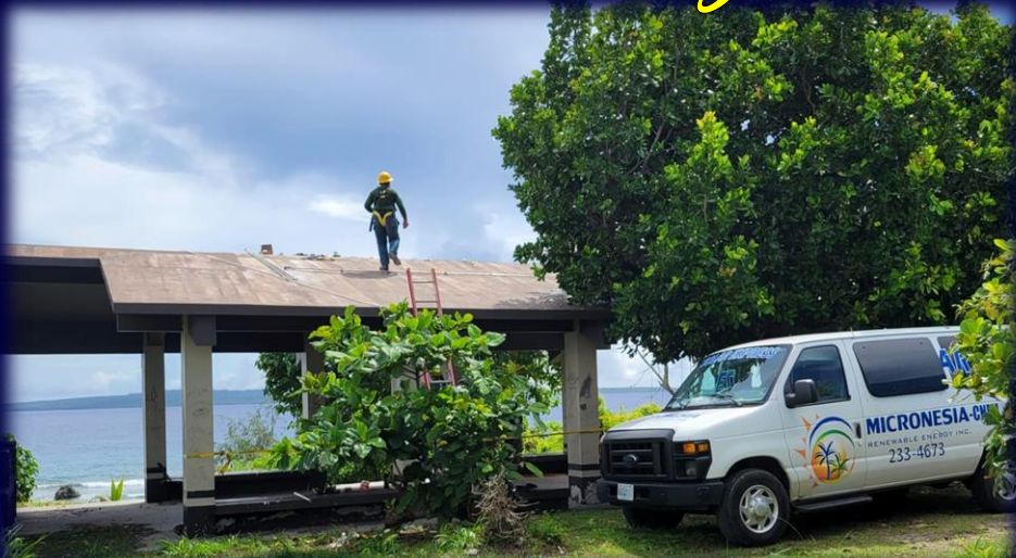
Solar PV Installation at Coral Ocean Point Beach Park – Saipan, MP 96950.
