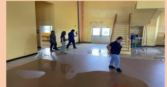
Heather Stole and her team during the inspection of the damaged Rota Gymnasium
